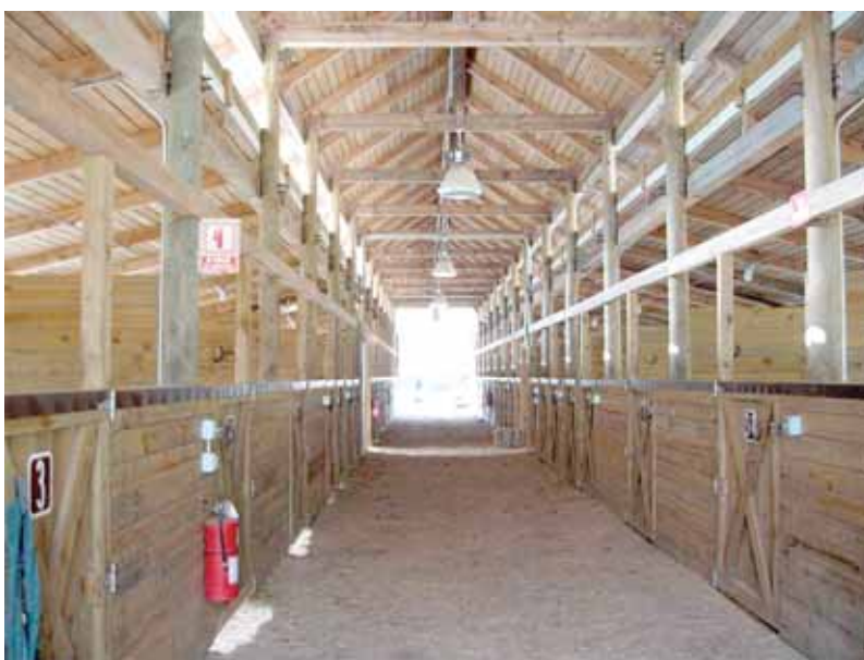
Fig. 9. The interior hallway of a well-constructed horse barn with post and beam. Note the safety features: all electrical in conduit, fire extinguishers, multiple exits, emergency lighting, ventilation, and easily opened latches. Photo courtesy of Tomas Gimenez.
