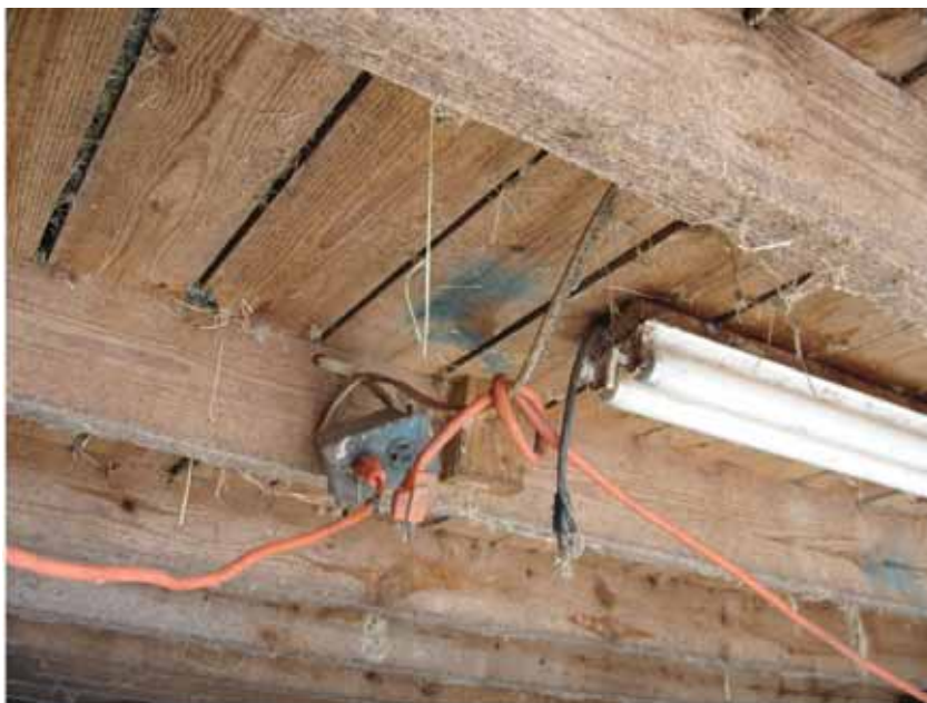
Fig. 14. Poorly designed and managed electrical service in a 12-stall horse barn. Photo courtesy of Tomas Gimenez.
