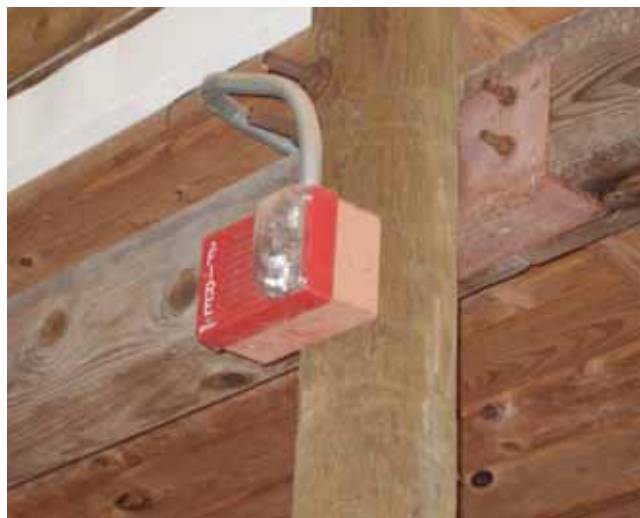
Fig. 6. Fire alarm siren and visual strobe light in conduit in a barn. Photo courtesy of Tomas Gimenez.
